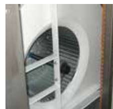
FAN GROUP WITH ANTI-CORROSION TREATMENT WITH SPECIAL PRIMER AND RAL 7035 GRAY COLOUR.
