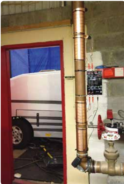
Vulcan S25 installed at Ice Land, New Jersey
