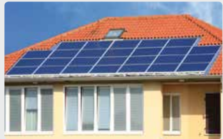
Solar heating panels on private house.
